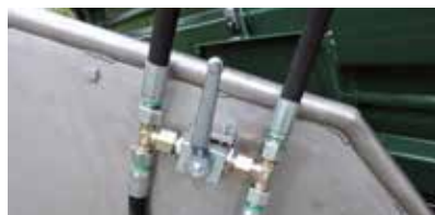
Shutdown via bypass
